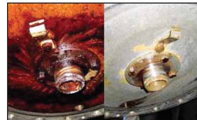
Vessel cover contaminated
